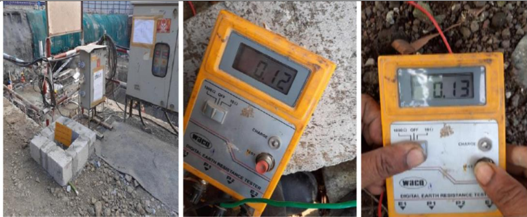
Certified Electrician, Approved SLD, Earth pit resistance display, Double earthing, and RCCB 30 mA protection
